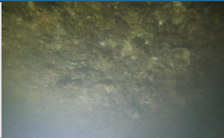
Image 2: Pile P-05 Below tide level covered largely by organisms.
